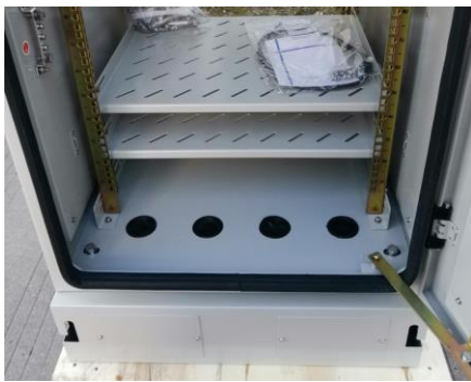
Cable entry, copper bars
